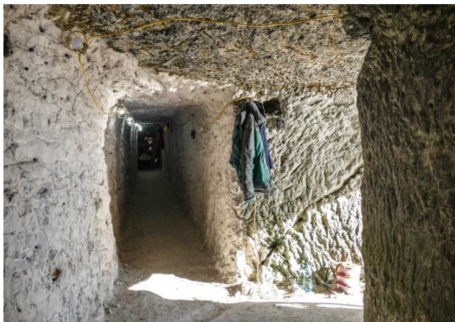
The new tunnel under construction in February 2019; to the right is the existing tunnel linking the searchlights to the location of the metal ladder to the beach, and behind the camera is the existing tunnel to the searchlight positions
